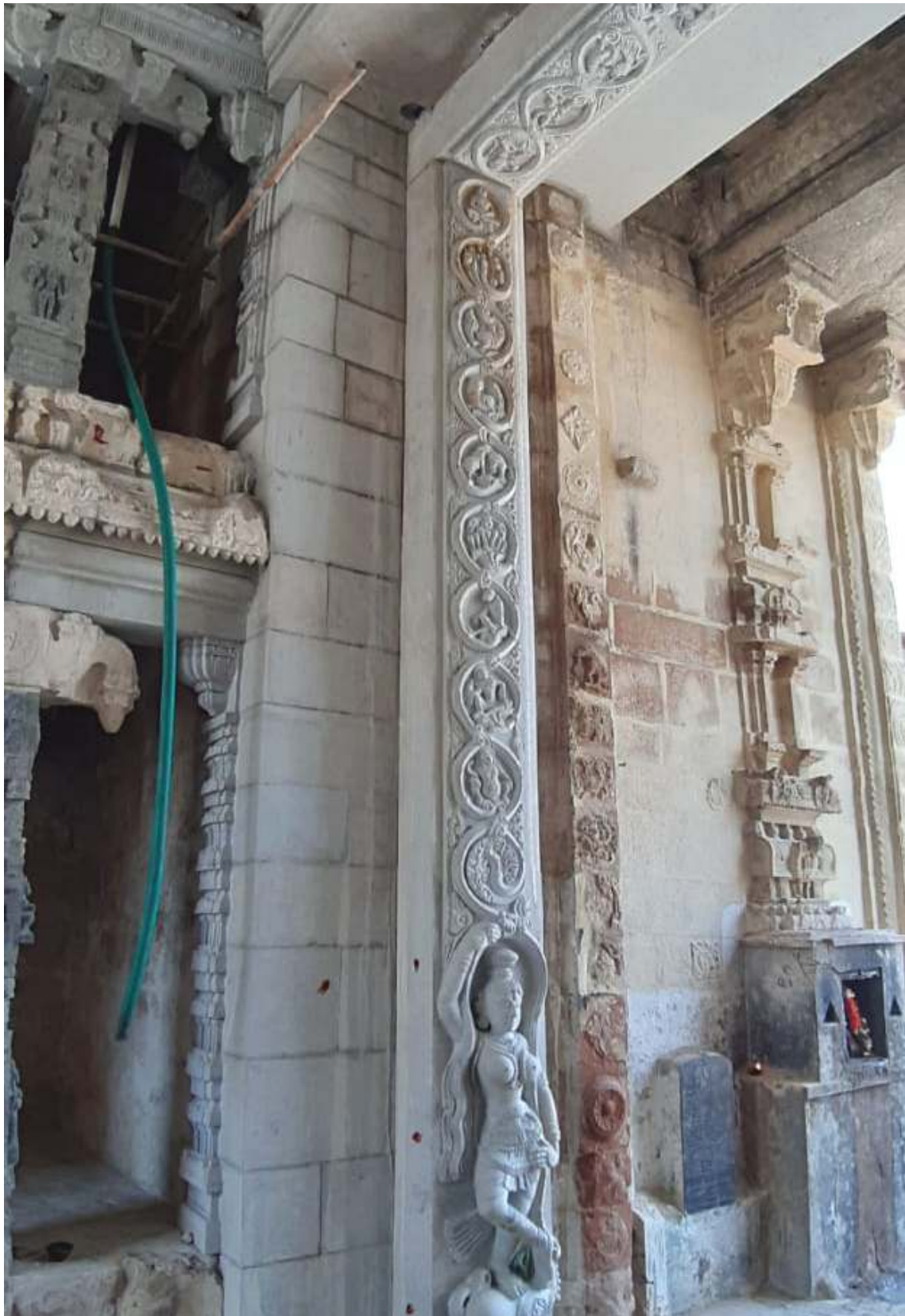
Shree Pundarikatcha Perumal Temple - Thiruvellarai The newly installed Door frame, RajaGopuram Entrance
