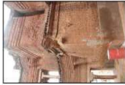
Figure 6: Deteriorated and abandoned masonry in upper floor
