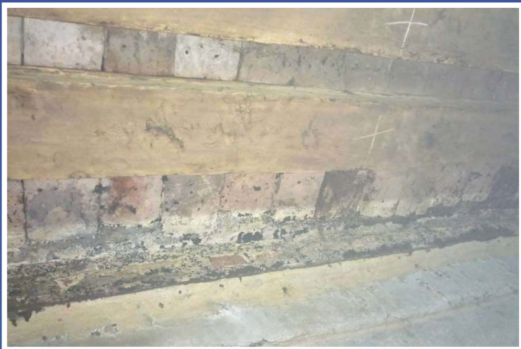
Deteriorated bricks ceiling in the sanctum santrum - May 2016
