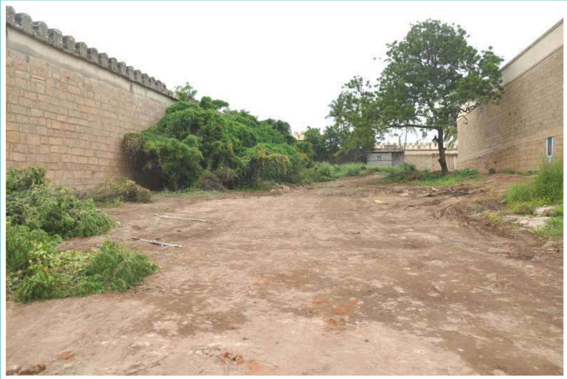
Too much of vegetation near the compound - Feb 2015
