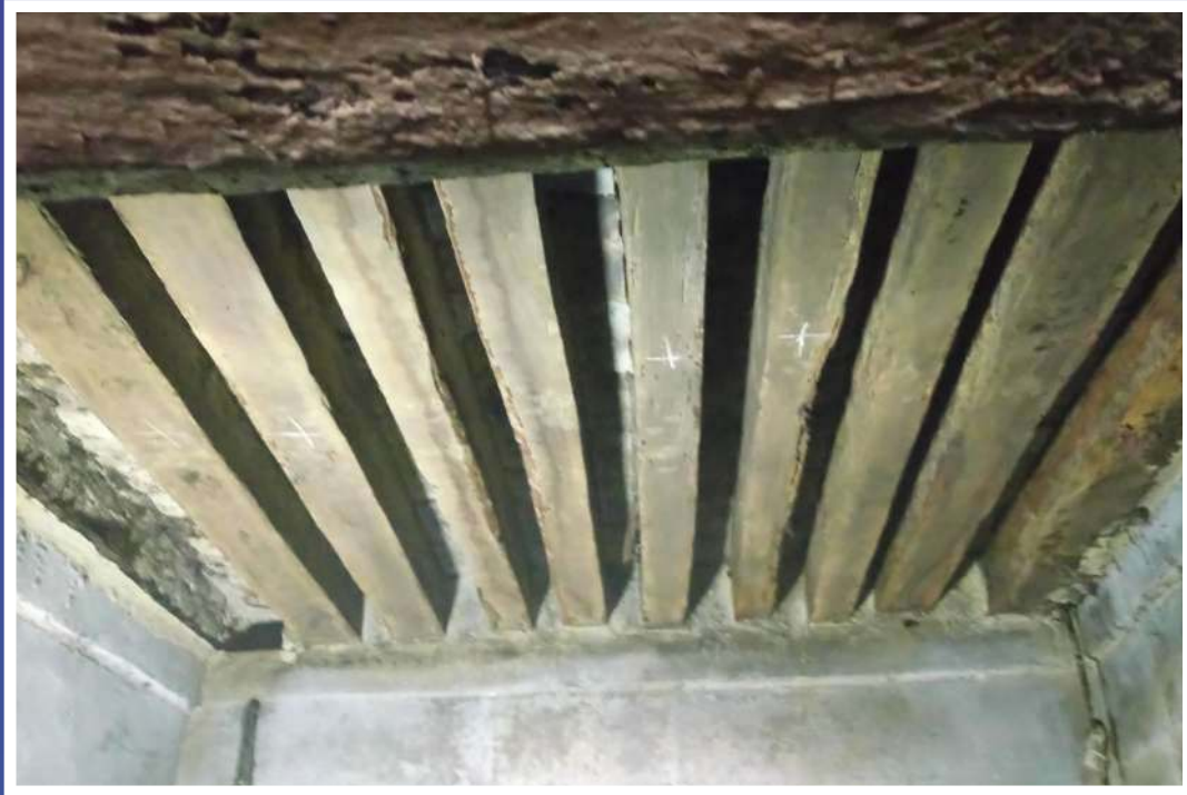
Deteriorated ceiling in the sanctum santrum - May 2016
