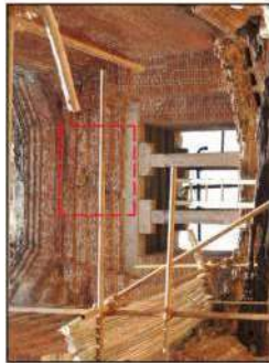
Figure 1: Deterioration in brick masonry; the second floor
