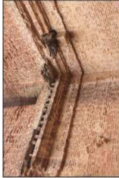
Figure 5: Deteriorated upper floor
