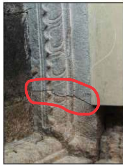
Figure 9: Cracks on granite beams
