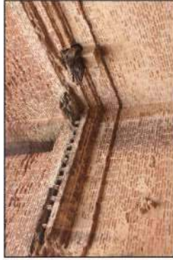
Figure 5: Deteriorated upper floor
