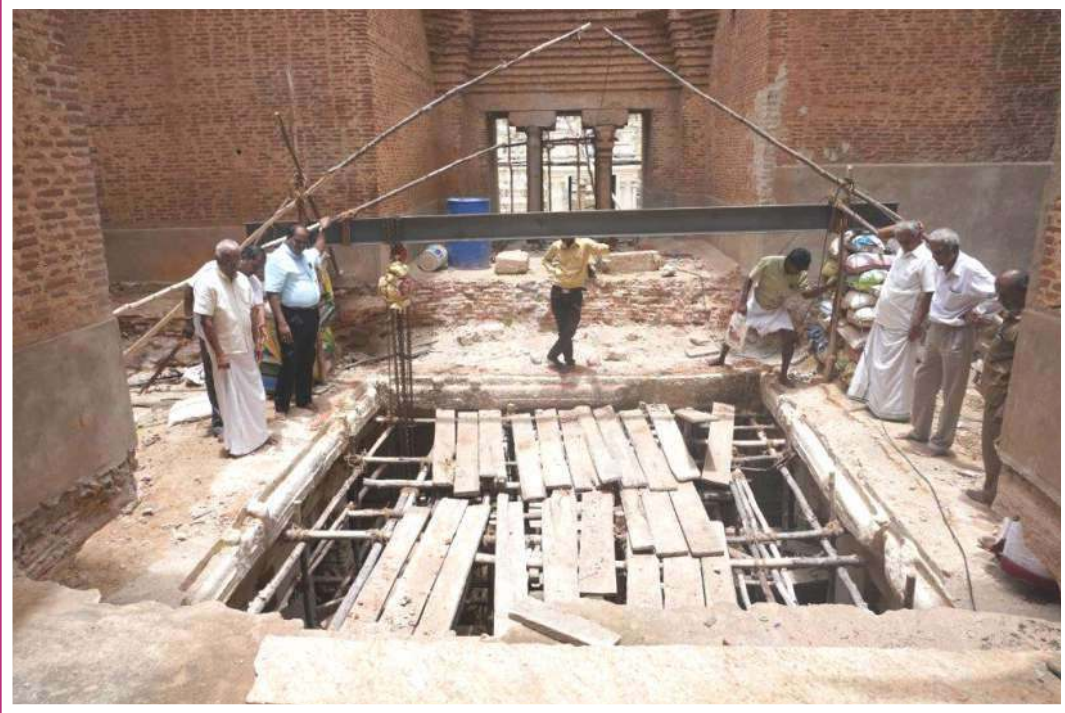
Joint Commissioner and the Donor inspecting the ground floor slab after being cut
