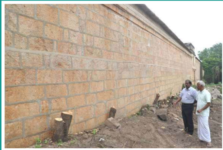
Huge trees have grown along the compound causing concern - Jan 2015 Sri Rangam Joint Commissioner Shri. P. Jayaraman inspecting
