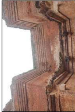
Figure 3: Deteriorated timber members
